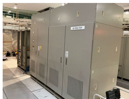
Figure 3. The new power supply for the bending magnets of the storage ring, manufactured by NICHICON CORPORATION.
