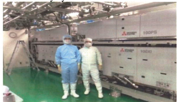
Fig.2 Pre-amplifier + 3x main amplifier installation by Mitsubishi Electric.
